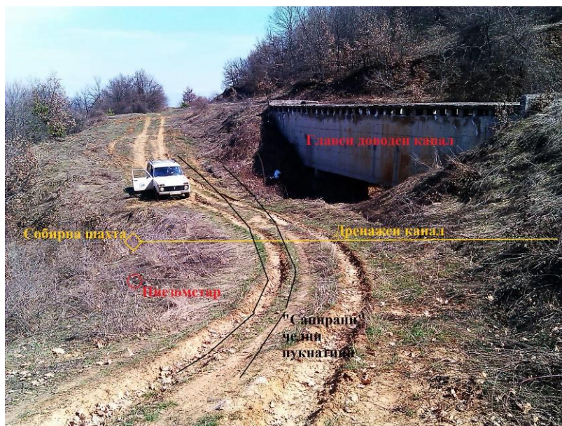
Figure 13. Current state of the landslide (source: photographed 29.03.2012)
