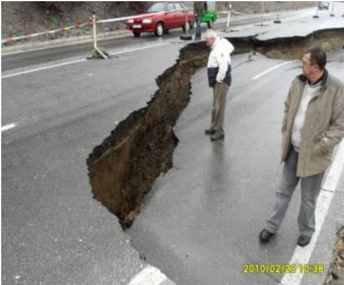
Landslide on the M-5 Resen-Bitola regional road, February 2010
