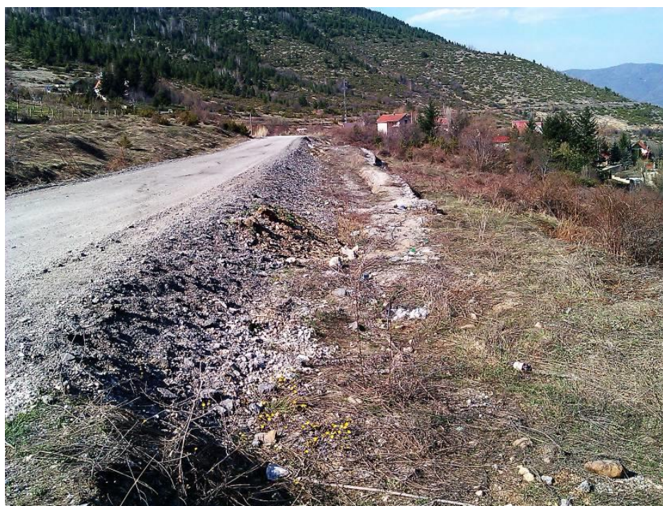
Figure 26. Location of support structure of gabions under the road Bitola - Nidze Pole (source: photographed 29.03.2012)
