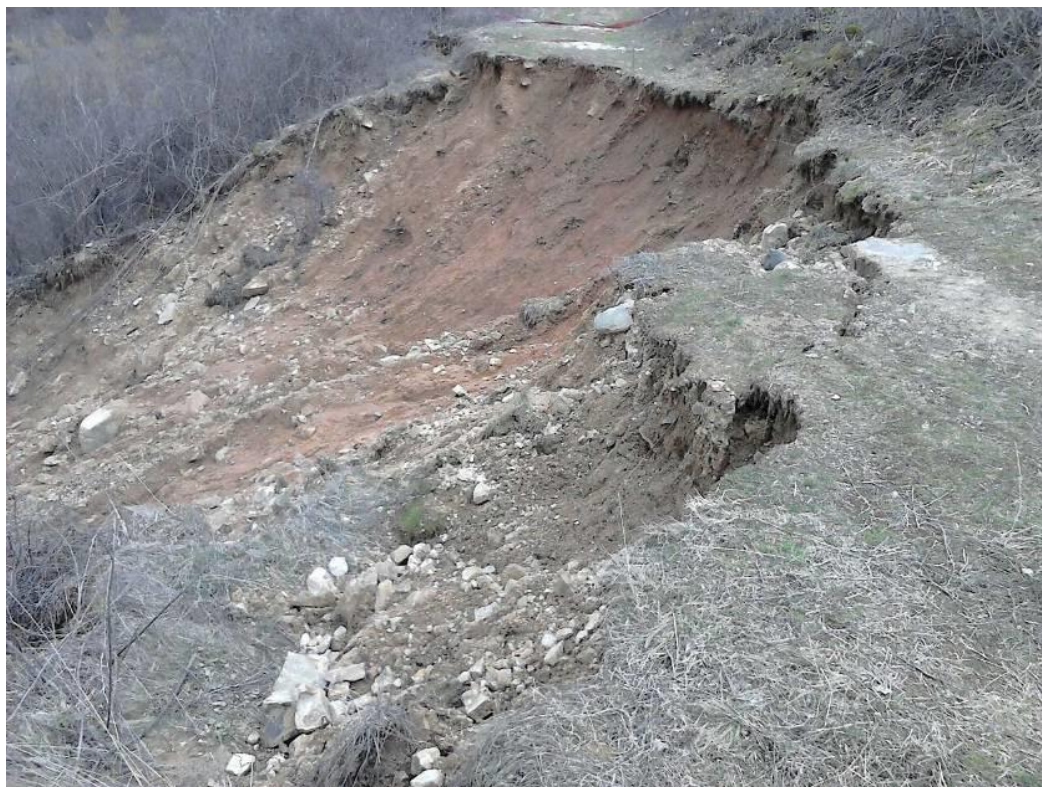
Landslides in the zone of the supply channel at Strezhevo hydro system
