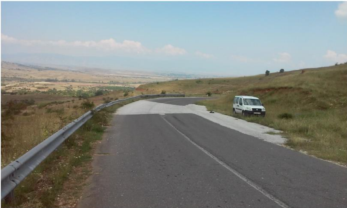
Figure 30. Landslide area adjacent to km 34 + 500
