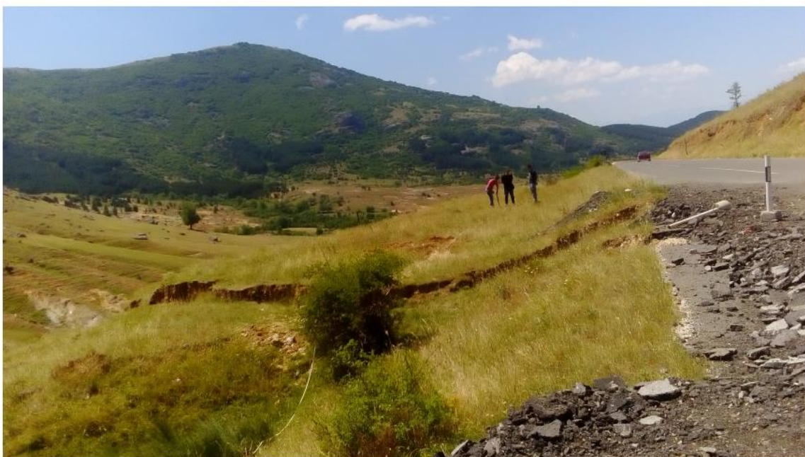
Figure 29. Landslide area just below the road at km 35 + 000
