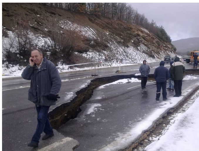
Figure 7. Frontal landslide fracture on 21.02.2010 with visible jump of about 0.6 meters and detachment of about 0.1 meters
