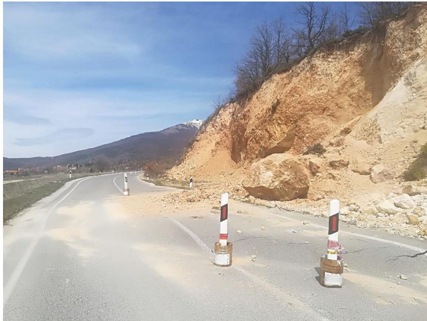
Figure 34. Photo of landslide on Pretor-Markova Noga road
