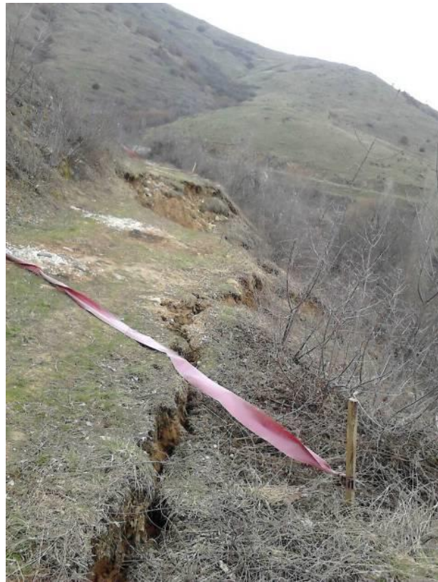
Landslides in the zone of the supply channel at Strezhevo hydro system
